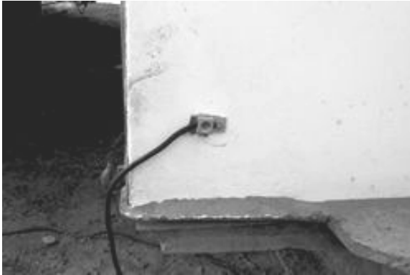
Note single metal-to-metal connection
